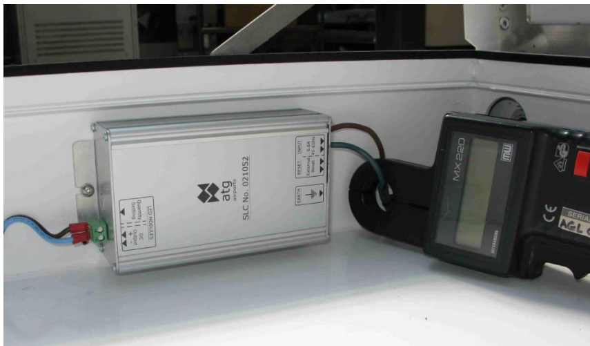
Figure 5.2 Open Circuit LED Fault Detection testing and reset
