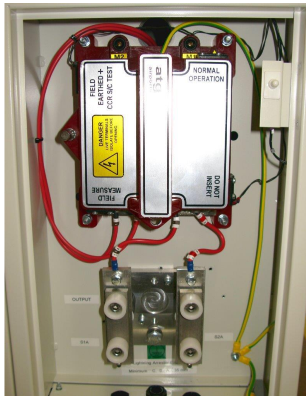
Figure 6-1 Cutout Switch mounted in CCR HT Output Terminal box
